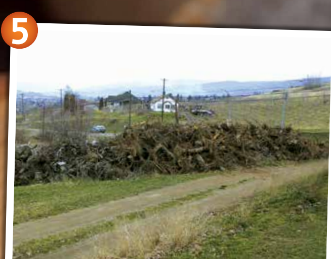
Step 5 Ensure the excavator makes one pile for every acre of trees pulled.
